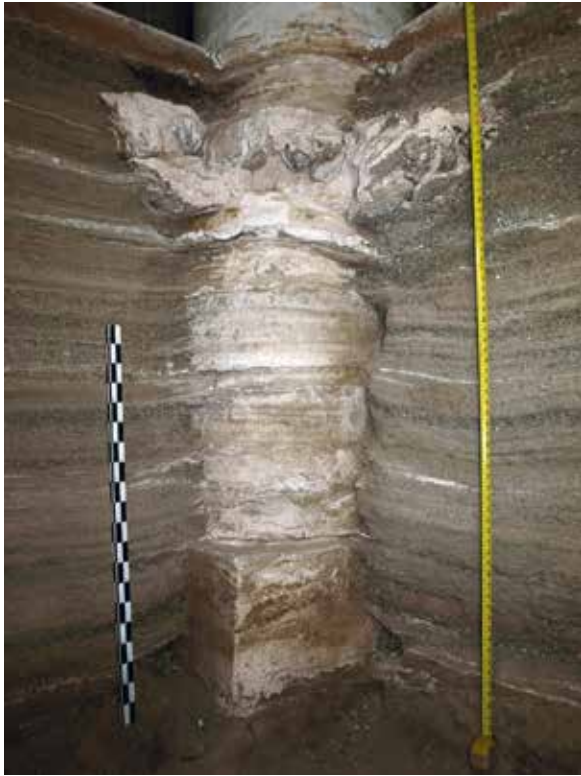
Fig. 31. Pillar E1 in the north riwāq . The ribbon foundation is visible at the bottom of the photograph. The original pier, with multiple replasterings, sits on a large plastered base. The present pillar is also a pier, established on a bed of large rough stones embedded upon the stub of the original pier.
