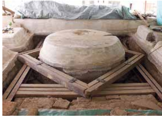
Fig. 18. Detail of part of the external wooden structure built to support the dome.
