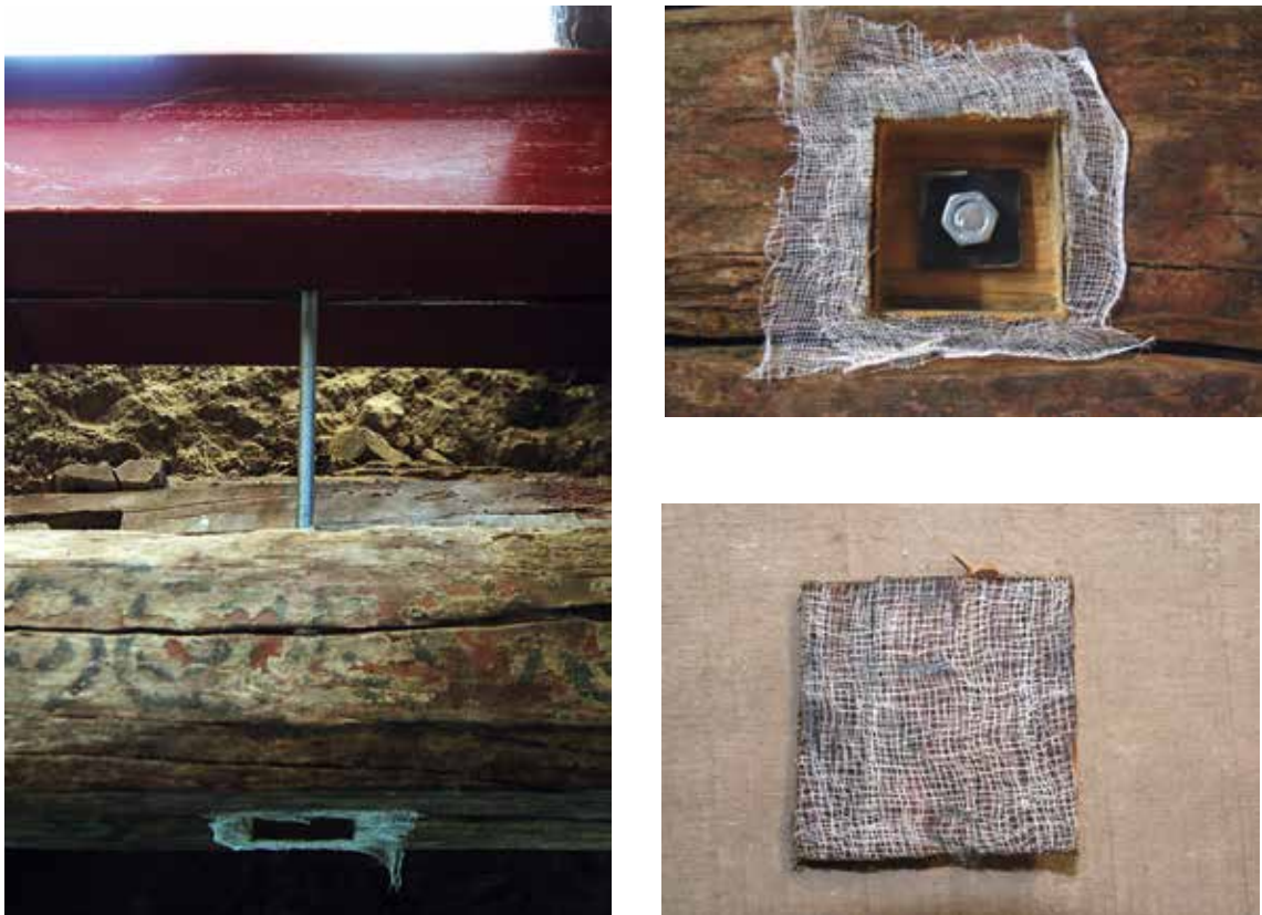
Figs 11, 12 and 13. Detail of the system used for inserting the hook bolt to the threaded tie rod.
