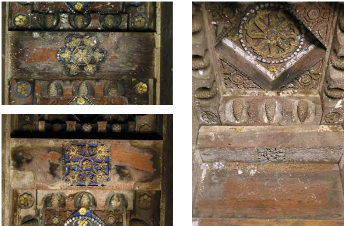
Figs 8, 9 and 10. Some examples of badly damaged coffered areas due to water seepage and percolation.
