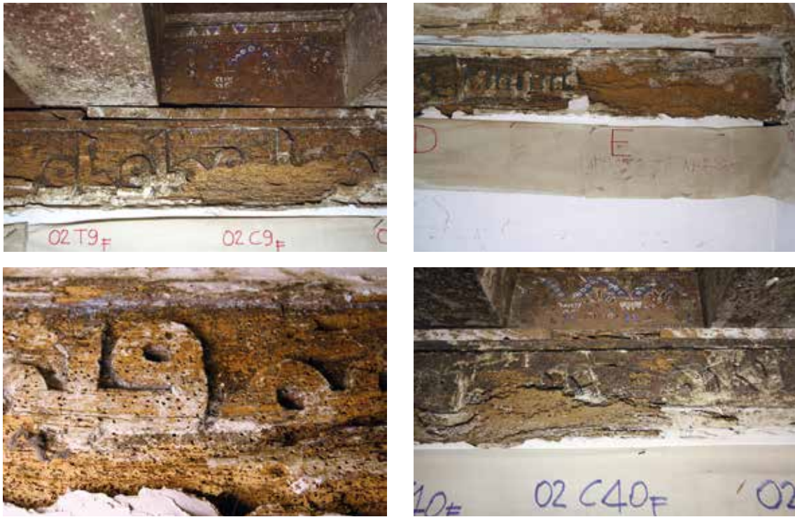
Figs 14, 15, 16 and 17. Details of the sleeper band obscured by the attack of xylophagous insects.
