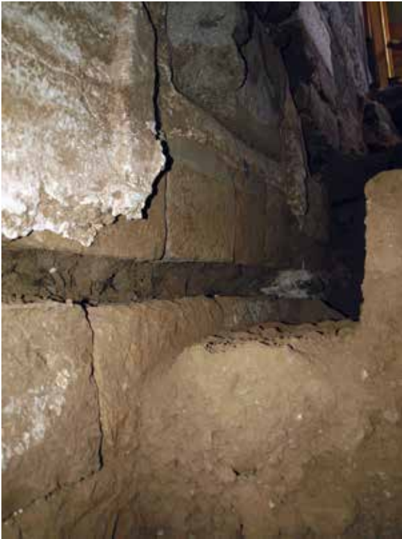
Fig. 21. Detail of the wood slot in the north face of the east minaret, below the original doorway (after removal of the stone step).
