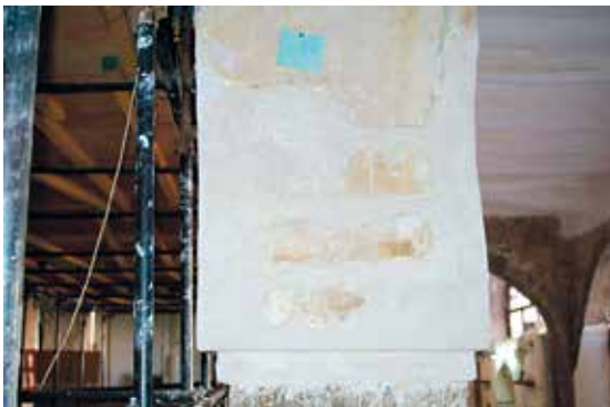
Fig. 79. Column no. 16 K, east side, application of plaster at the base before the final layer.
