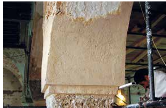
Fig. 80. Column no. 16 K, west side, application of base coat in preparation for final plastering.
