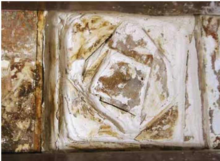
Fig. 23. Example of an old maintenance operation where the coffer probably covered with plaster to fix and stabilize its unsafe elements.
