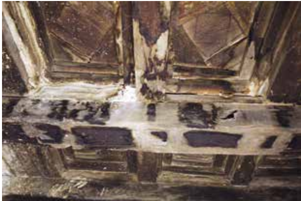
Fig. 18. One of the largest areas in which rainwater, seeping in from the ceiling, washed the decorated surfaces off the ceiling.
