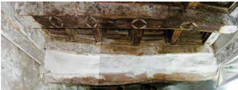
Fig. 2. Example of one of the most common types of maintenance work performed in the past to solve the problem of a fractured beam at risk of collapse.
