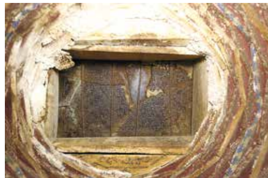
Fig. 10. Details of the skylight of the SW dome. Also in this case, in an attempt to restore the wooden structure, large plaster walls were built which over time which had become unsafe and at risk of collapsing.
