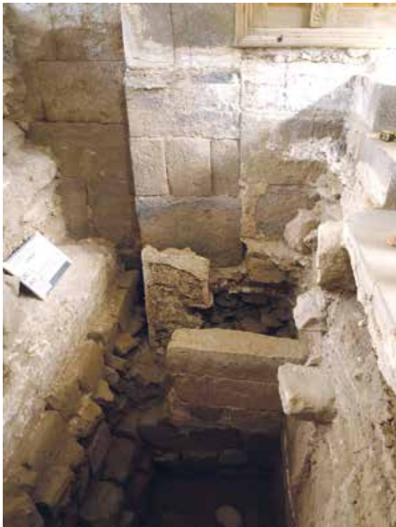
Fig. 2. Exterior face of the north wall, the surround of the imam's doorway, and remains of the earlier formal entryway. Note the large size of the facing blocks of the wall.
