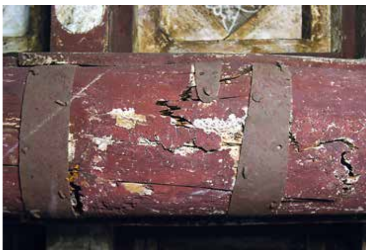
Fig. 21. Example of an old maintenance intervention that attempted to repair or avoid a complete fracture of the beam.
