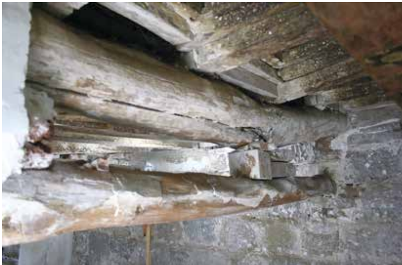
Figs 3, 4 and 5. Some examples of borderline situations of transversely fractured beams and the related past repair attempts.
