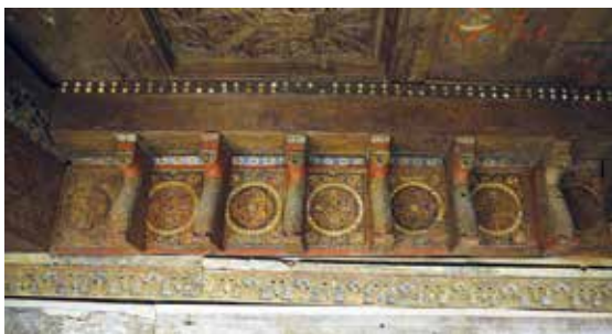
Figs 38, 39 and 40. Top: two details of the lateral decorations prior to restoration. On the left a detail of the decoration after restoration.
