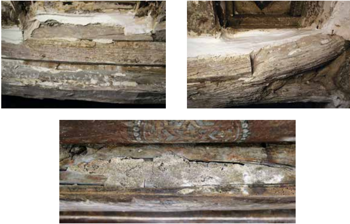
Figs 48, 49 and 50. Beams and coffers with wooden or brick and plaster infill to fill in the gaps or the loss of original wooden elements.
