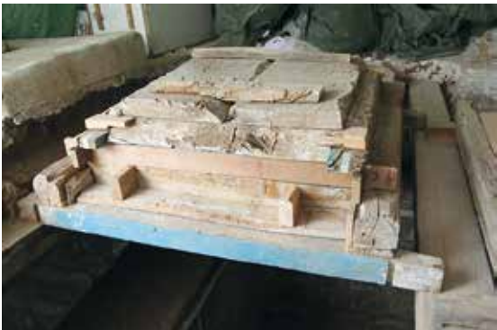
Fig. 18. Phase of the structural intervention in an intermediate stage of reassembly of the upper cap.
