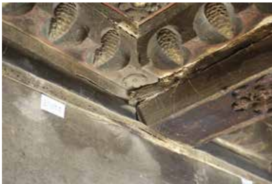
Figs 5, 6 and 7. The photos highlight typical situations of deterioration of the eastern riwāq , in particular the attack of xylophageous insects on the narrow frames that divide the elements of the coffers.
