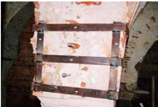
Fig. 89. Column no. 17 K, north side, patching of gaps with hydraulic lime and application of metal cage.
