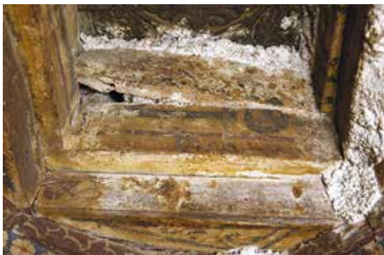
Fig. 9. Details of the skylight of the NW dome which highlights the precarious state of conservation. The wooden boards showed serious disconnections and large plaster infills.
