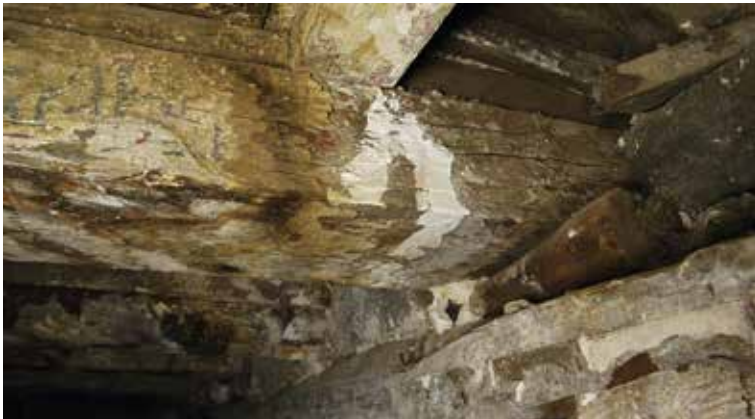
Fig 47. Cracked and/or remodeled beams, incorrectly and unsafe inserted in the masonry, and supported on the side only by wooden and / or brick shelves.
