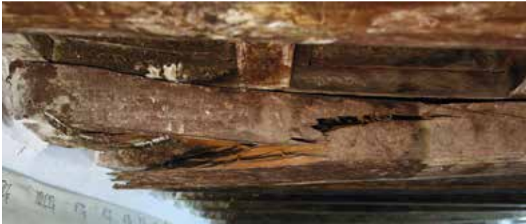
Fig. 45. Beams with large cracks and transverse fractures with relative static and structural weakening.
