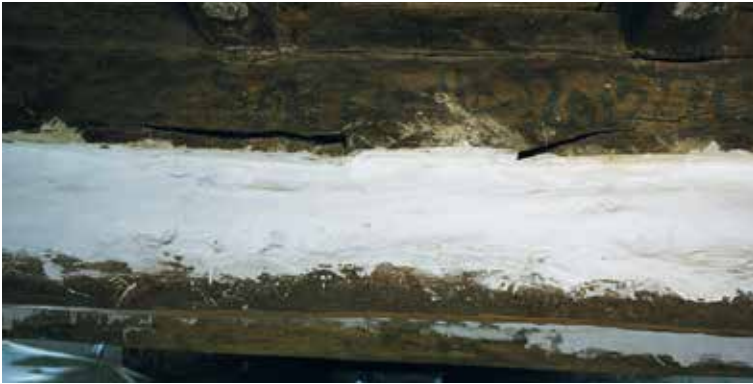
Fig. 42. Crosswise fractured beams supported by an additional support beam, generally an unworked and rather rough wooden beam, with a circular section added in the lower part and the heads set in the masonry. The large empty space between the two beams was filled with plaster and brick infill.
