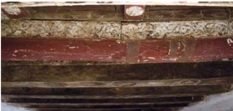
Fig. 46. Beams with large cracks and transverse fractures and related old restoration intervention consisting of metal elements of the most varied type (hooks, nails, chains, pulleys, etc.)
