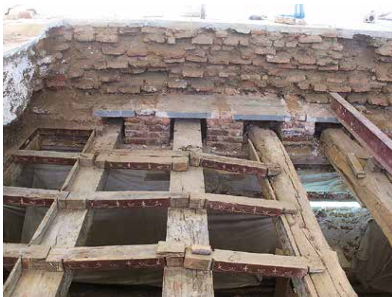
Fig. 7. The dismantled coffered beam and joist system is visible in the image.
